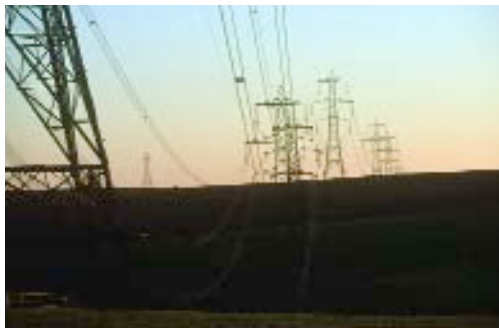
Intrusive elements degrade the landscape.
