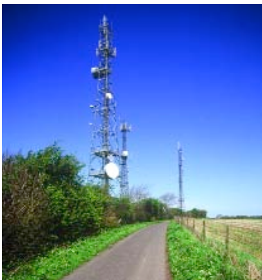
Communication masts, signs and other infrastructure along roads impact on the AONB landscape.
