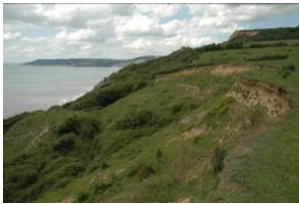
Coastal erosion is an issue which needs to be increasingly addressed
